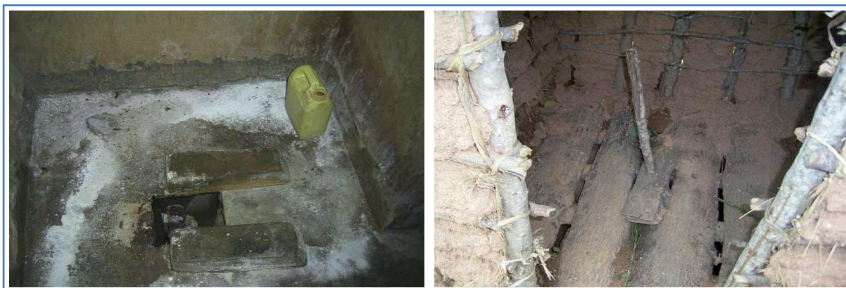
Figure 5: Latrine with cement base and washing water, Rusumo (left) and wooden latrine, Umuyange (right) Source: Mareile Zöllner
