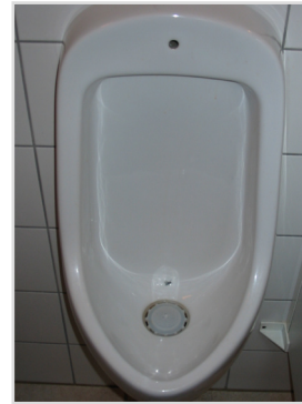
Figure 2: Waterless urinal (Source: A. Rechenburg)
