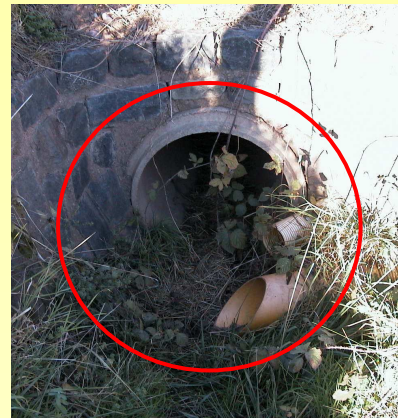
Photo 2: Drainage pipes at the Suerstbach
